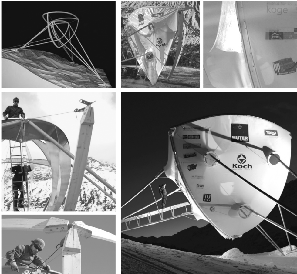
Figure 8 Full scale Case Study 01, Documentation of the assembly, Nov. 2014, Above left static concept model in 1:50
