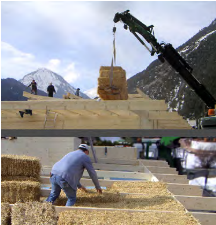
Pic.8 Haus Schönwies, insulation with straw, Tyrol 2006, foto by w. Kłasz, design and supervision by w. Kłasz
